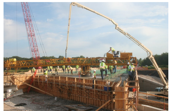
Crews pour the concrete for the Gutermuth Road bridge deck on August 15, 2013.
