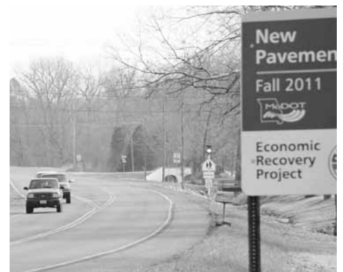
Major improvements to Route 34 from Piedmont to Silva were completed ahead of schedule. The project was expected to be completed in fall 2011. Minor bridge work will be completed this spring.
