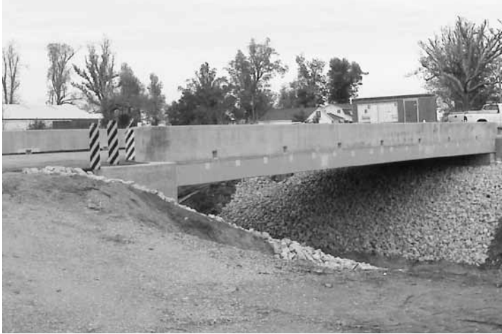
The opening of the Route 153 bridge over Drainage Ditch No. 7 in New Madrid County marks D10's halfway point in the Safe & Sound program.
