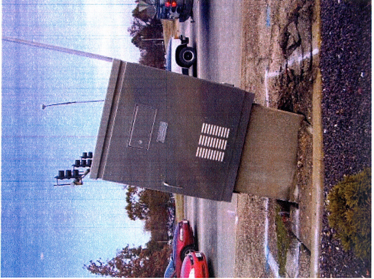
Slide 4- Existing Damaged Base
