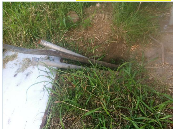
Buried Conduit/Wires Facing Street Lights on I-70
