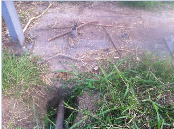
Buried Conduit/Wires Facing Power Source Pole
