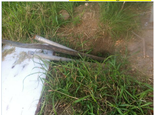
Buried Conduit/Wires Facing Street Lights on I-70
