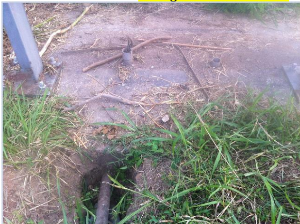
Buried Conduit/Wires Facing Power Source Pole
