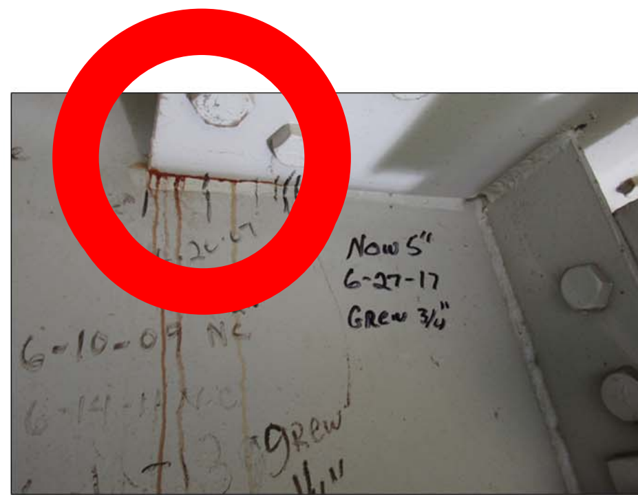
Some of the steel connections are cracking apart.
