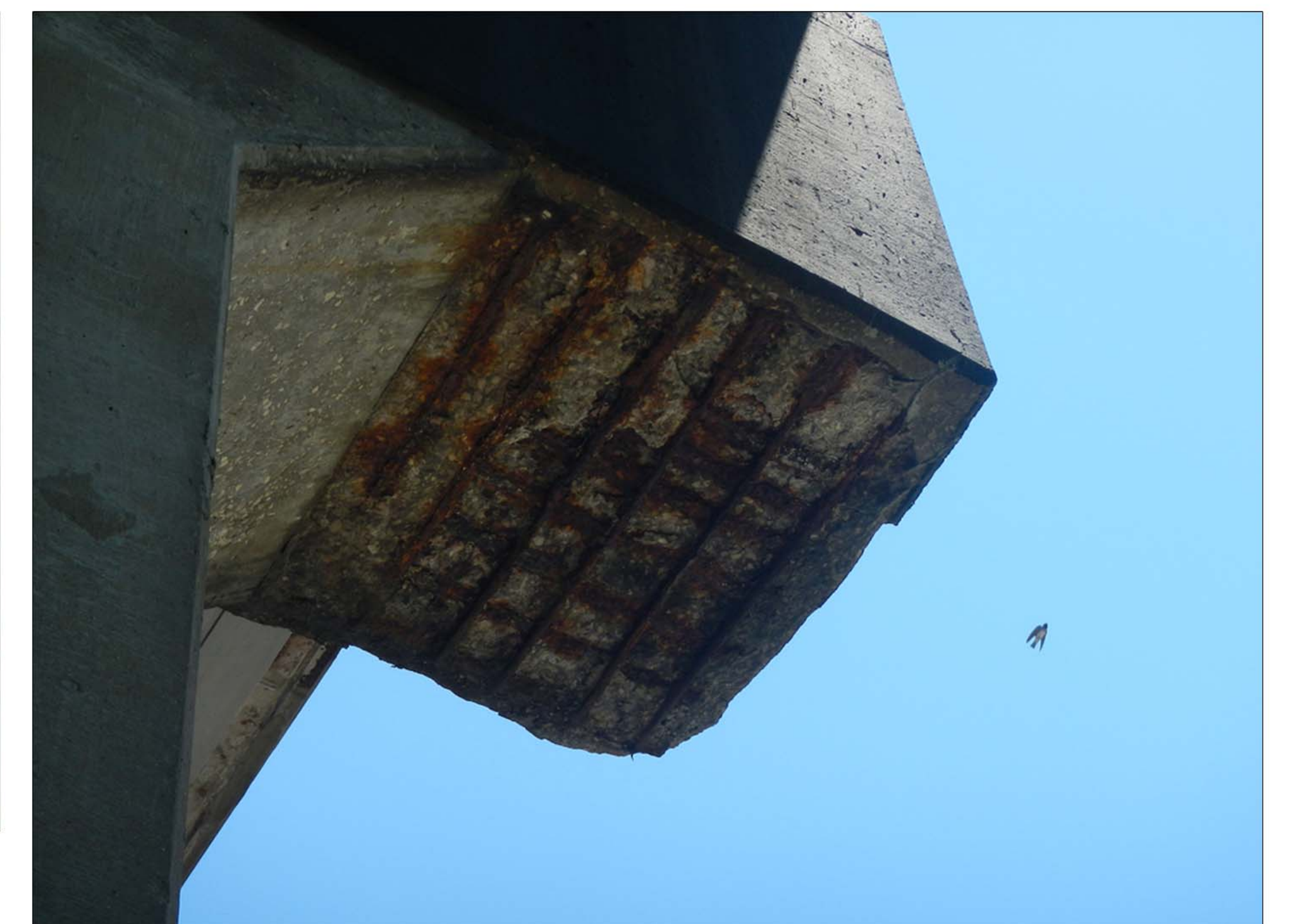
Portions of the reinforcing steel are exposed and rusting.
