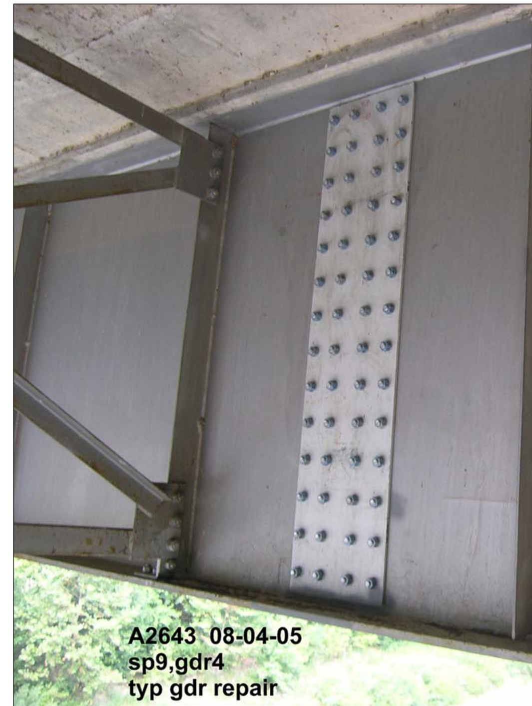
The plate here helps strengthen an area where the girder is weaker.
