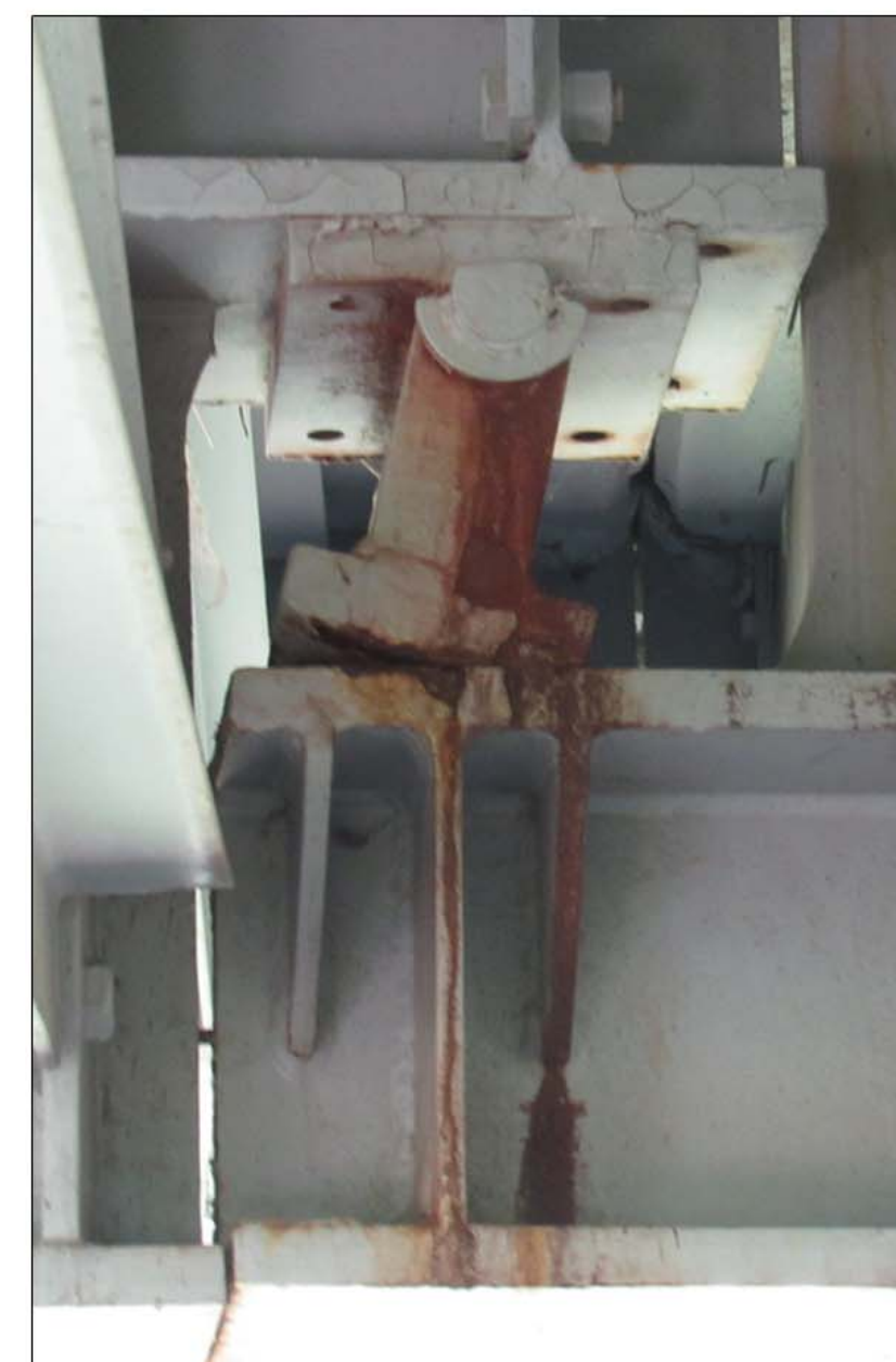
This piece helps ensure the bridge can move as the bridge heats and cools. It is rusted and stuck.
