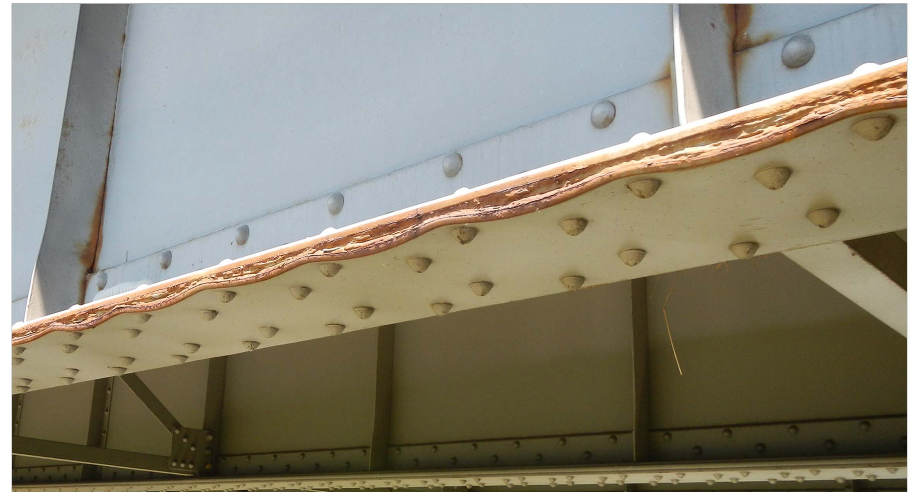
Bridge girders are starting to rust and deteriorate.
