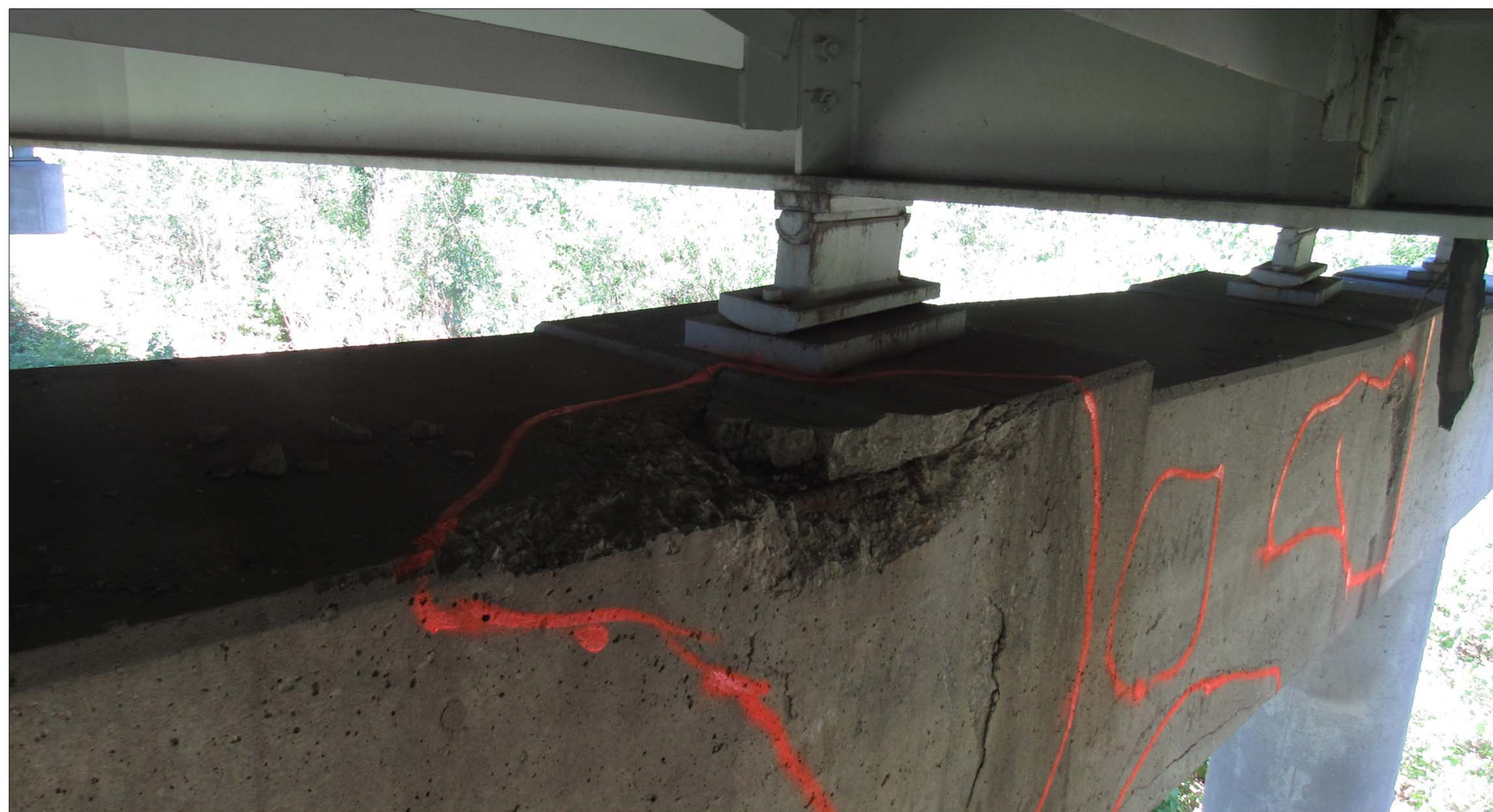
The concrete foundations are cracking and crumbling.
