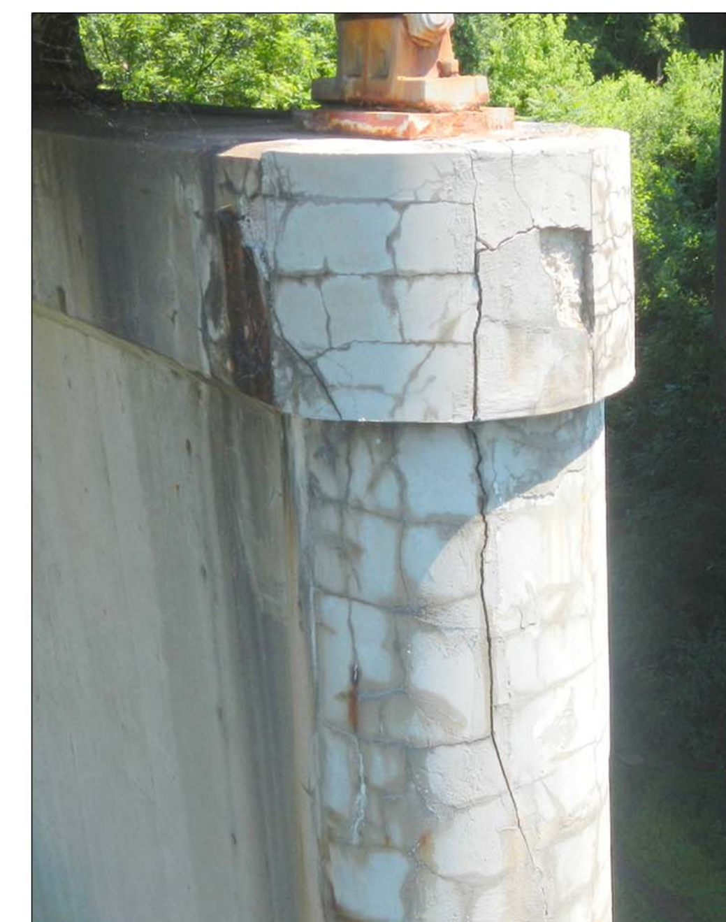
Concrete in the foundation is starting to wear out and crumble.
