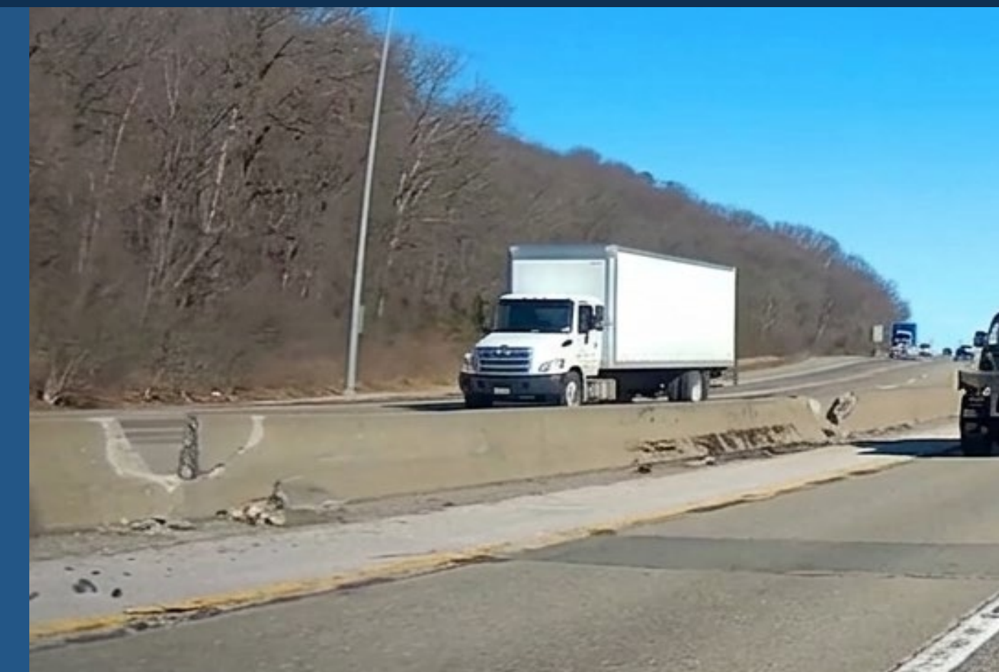
Damaged Median Barrier
