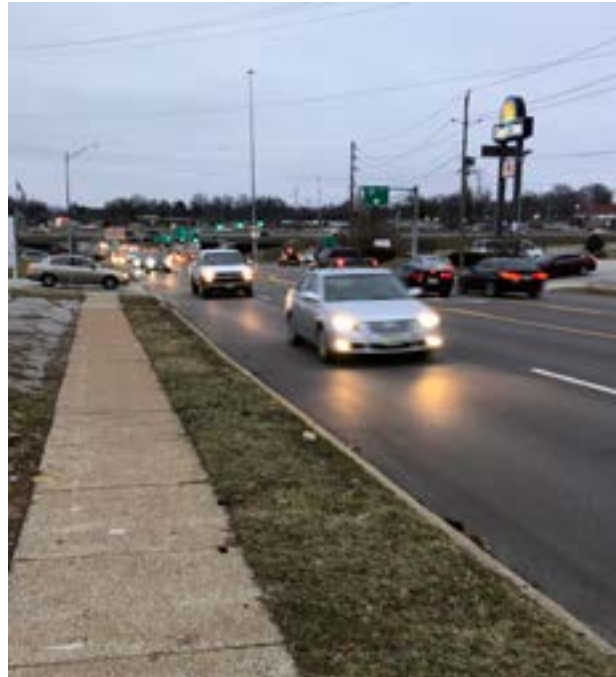
North Hanley Road Resurfacing - Working with the St. Louis County Department of Transportation, Oates resurfaced North Hanley Road, a heavily travelled roadway that connects to three major highways and access to several major employers. This project improved the driving surface while integrating safety for all modes of transportation - including upgrading the pedestrian realm to be ADA compliant.
