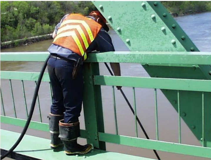
Spring and fall flushing should include all bridge items, drains system, drain basins, and under expansion devices.
