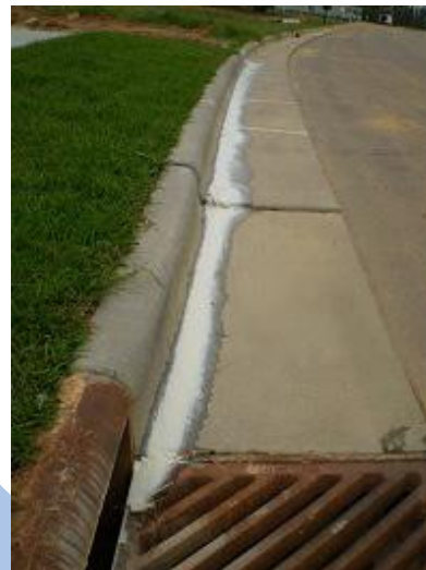
Evidence of an Illicit Discharge
