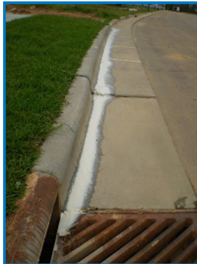
Evidence of an Illicit Discharge
