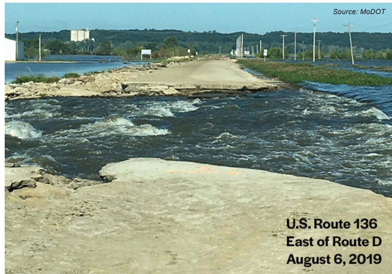
Figure 38 – 2019 Flooding Washes Out a Section of U.S. Route 136
