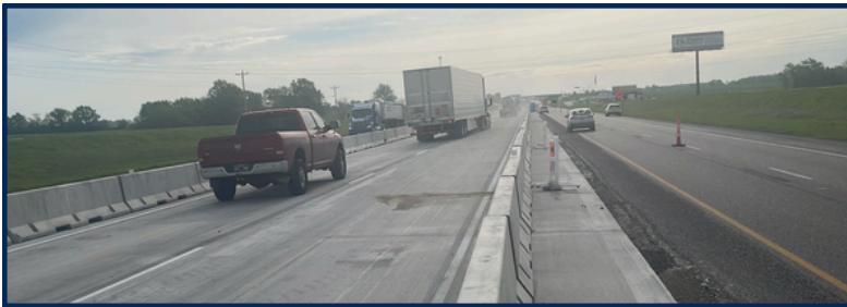
Crews have switched traffic along eastbound I-70 onto new pavement between Callaway County Routes J and M.
