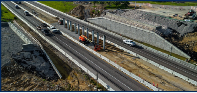
Progress continues on the new MO Route 47 bridge over I-70 in Warrenton.
