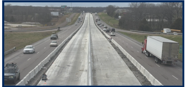
Paving of the third lane of I-70 continues between Callaway County Routes J and M.
