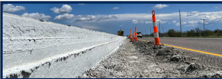
New pavement on I-70 between Callaway County Routes J and M compared to existing lanes.
