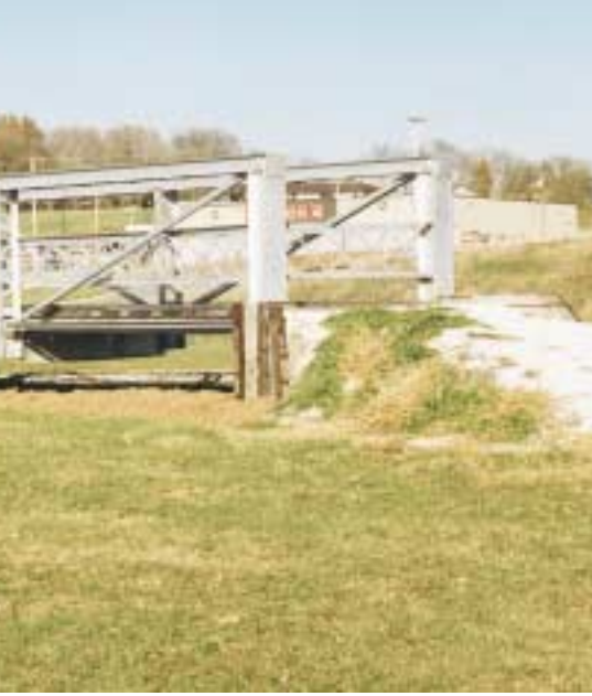
This 15-foot bridge in Carroll County is one of the smallest structures saved by the program.
