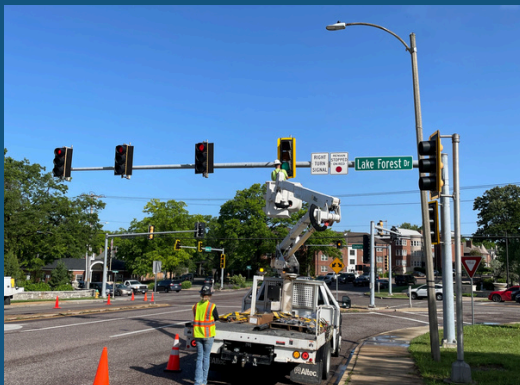
Retroreflective signal backplates replaced at signal -Lake Forest & Hanley Road Intersection - Richmond Heights, MO
