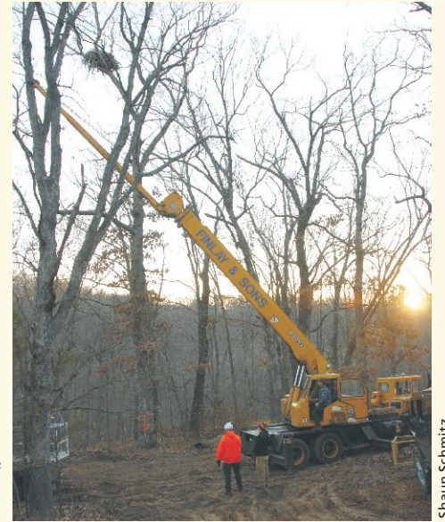
It took a crane borrowed from the contractor to remove the nest, which was about 50 feet up in the tree. The nest removal took about an hour.
