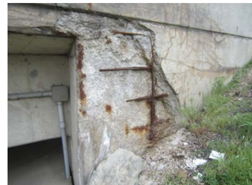
Figure 21. Spall with exposed reinforcing steel
