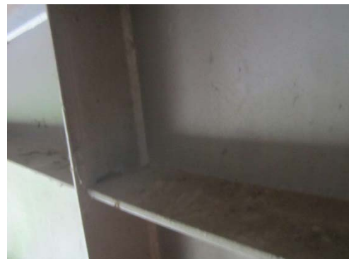
Figure 5. Small or missing gap at longitudinal stiffener
