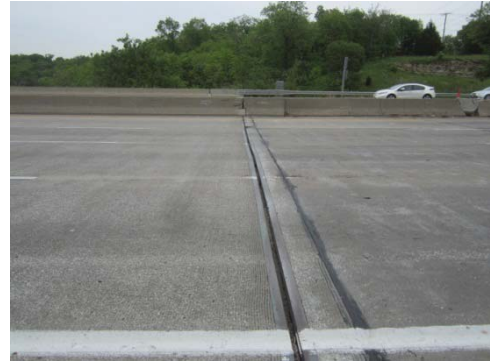
Figure 7. Deterioration in east abutment joint
