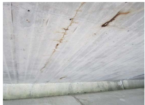
Figure 17. Cracks and rust stains on bottom of deck
