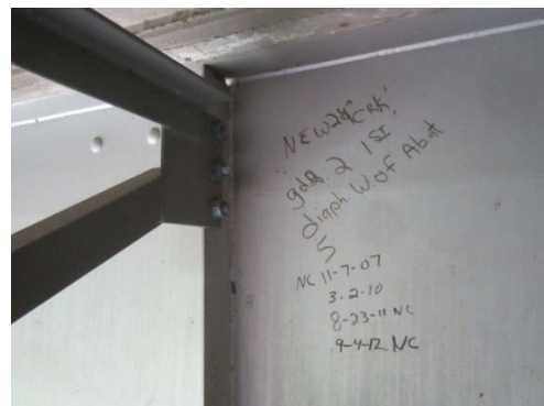
Figure 4. Typical crack in girder web
