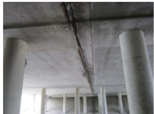
Figure 16. Spalls along longitudinal joint
