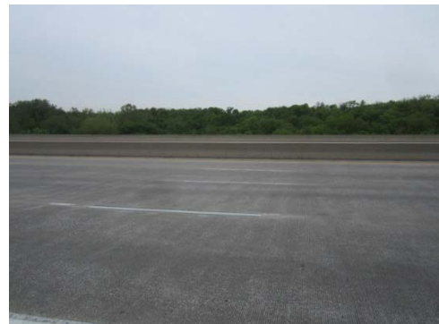
Figure 8. Cracks in median barrier
