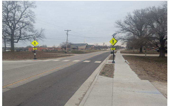
Bartlett & West provided complete construction phase services for the N Summit Drive improvement project in the City of Holts Summit.
