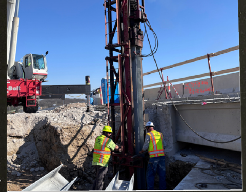
Crews driving bridge pile on the northbound U.S. Route 63 bridge over Conley Road.
