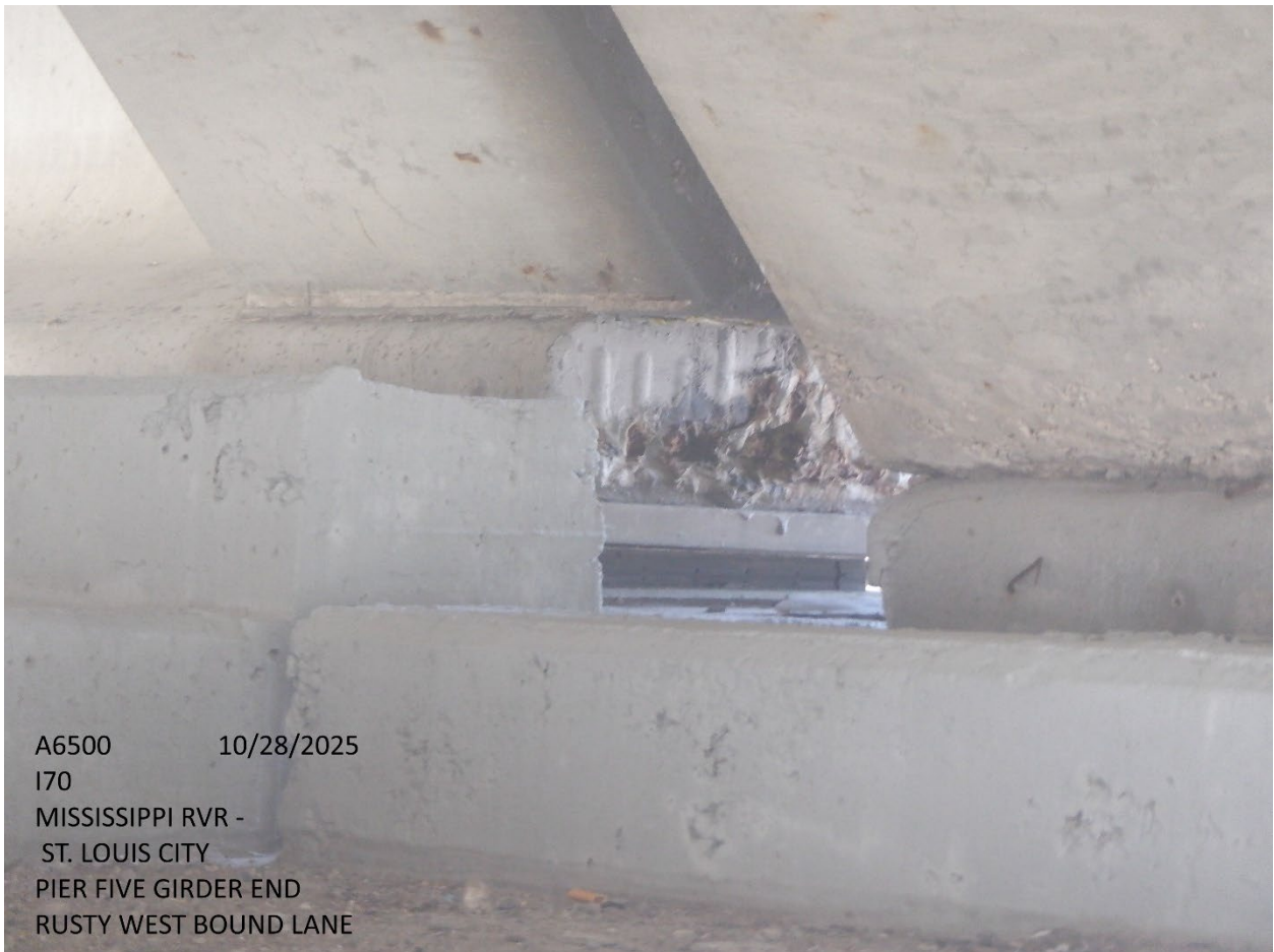
A6500 10/28/2025 I70 MISSISSIPPI RVR - ST. LOUIS CITY PIER FIVE GIRDER END RUSTY WEST BOUND LANE
