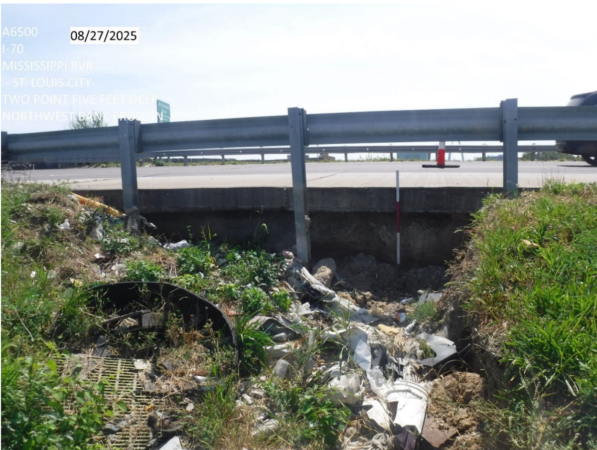
A6500 08/27/2025 I-70 MISSISSIPPI RVR - ST. LOUIS CITY NORTHWEST BANK EROSION TWO FEET UNDERMINING
