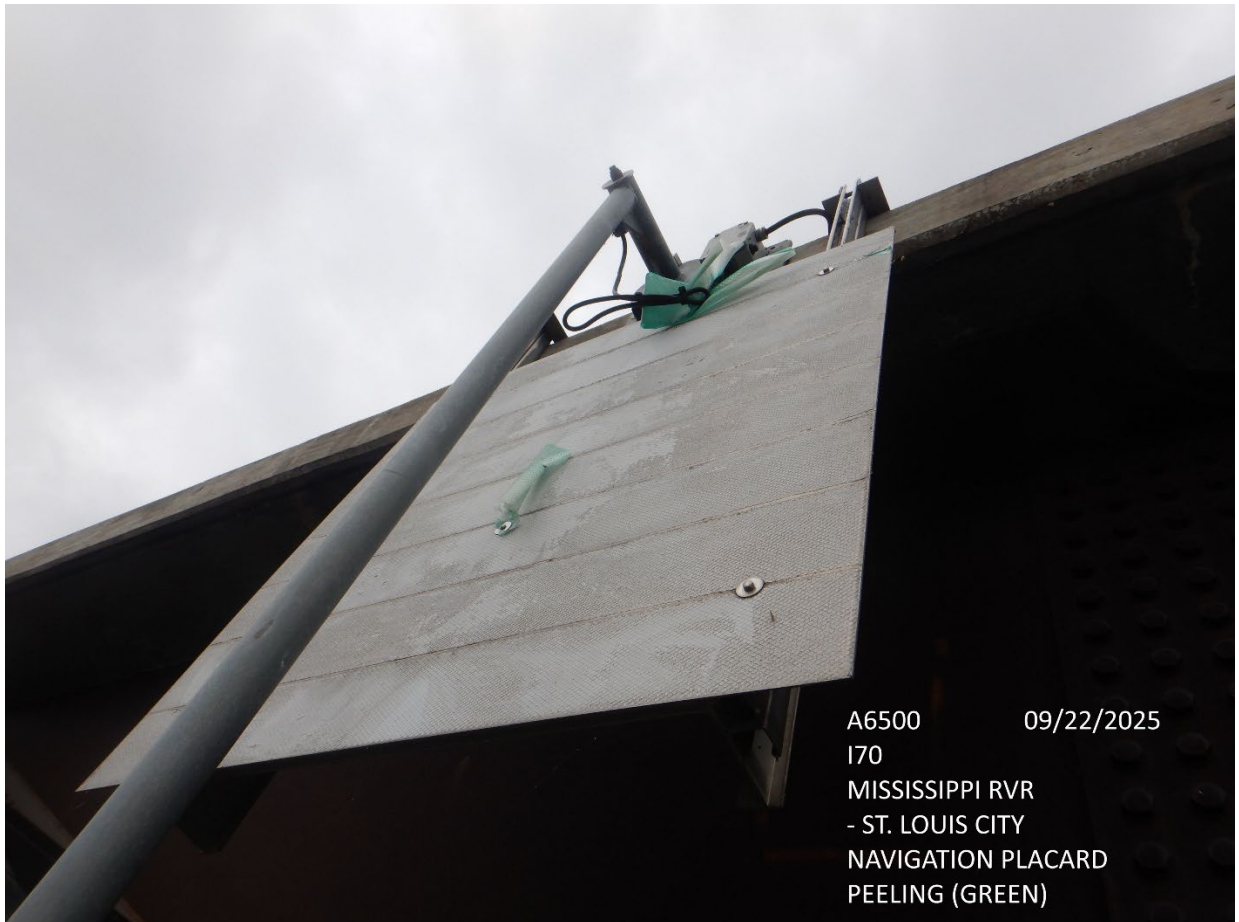
A6500 09/22/2025 I70 MISSISSIPPI RVR - ST. LOUIS CITY RED NAVIGATION PEELING
