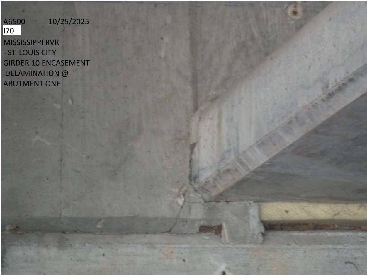
A6500 10/25/2025 I70 MISSISSIPPI RVR - ST. LOUIS CITY DIAGONAL CRACK IN GIRDER ONE SPAN ONE WITH/EFFLORESCENCE
