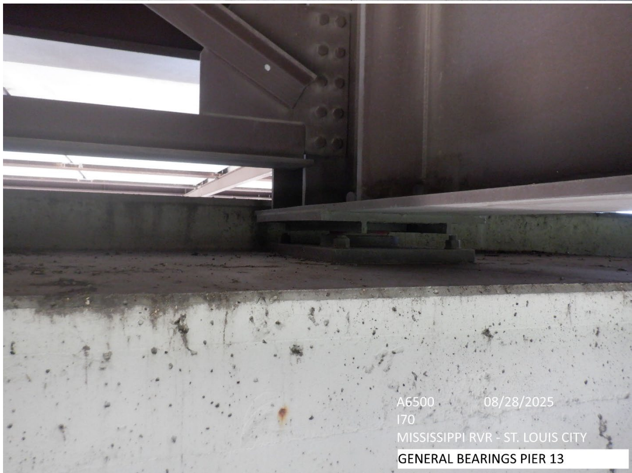
A6500 08/28/2025 I70 MISSISSIPPI RVR - ST. LOUIS CITY PAINT PEELING EAST SIDE OF PIER 13
