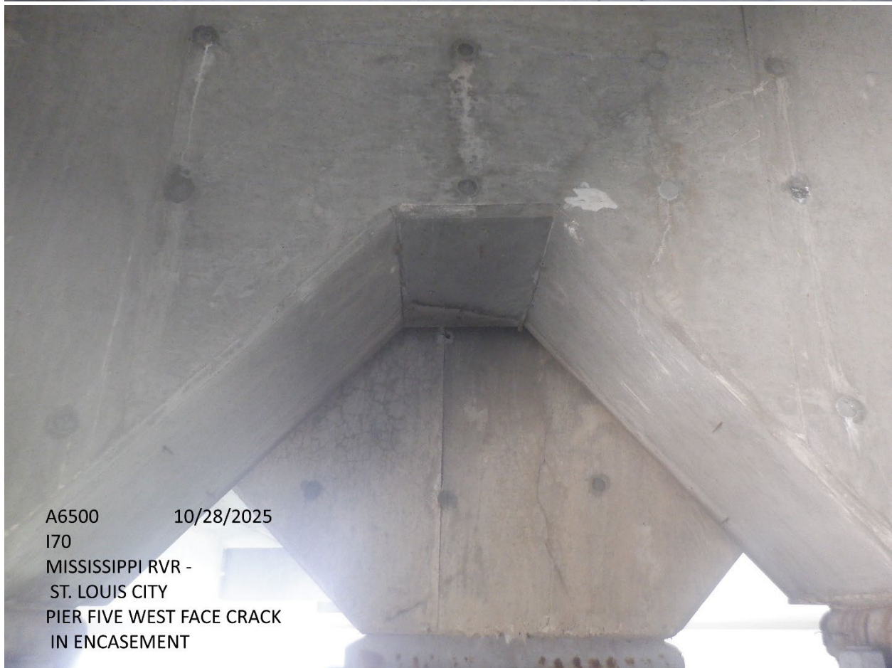
A6500 10/28/2025 I70 MISSISSIPPI RVR - ST. LOUIS CITY WEST FACE RUST ON SOLE PLATE @ PIER FIVE
