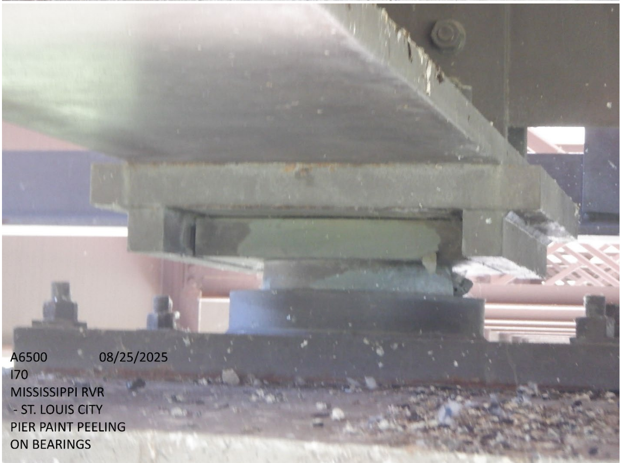
A6500 08/25/2025 I70 MISSISSIPPI RVR - ST. LOUIS CITY RUSTING BEARING PLATE @ PIER SOUTH END
