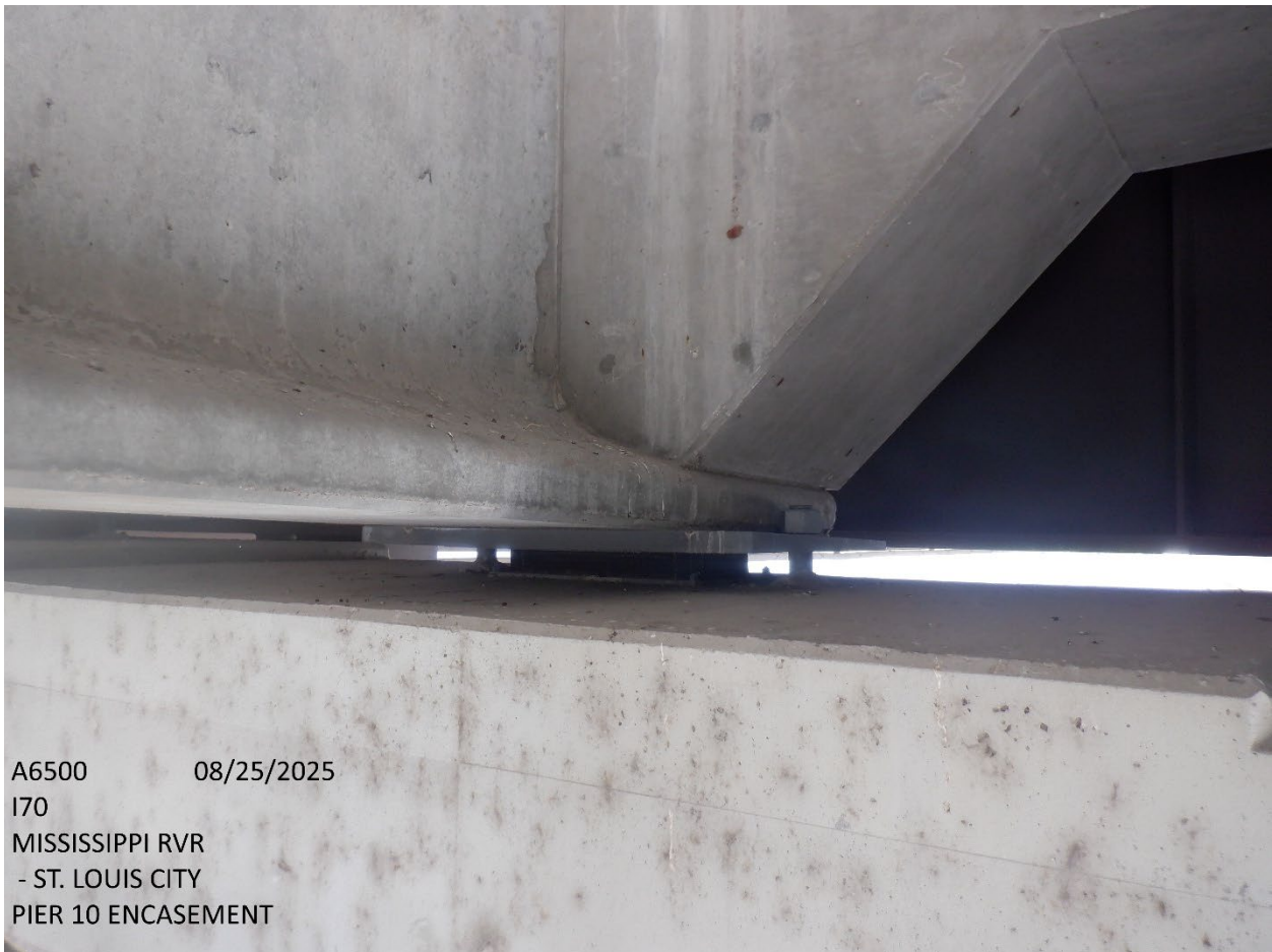
A6500 08/25/2025 I70 MISSISSIPPI RVR - ST. LOUIS CITY PIER 10 CHIPPED GIRDSERS
