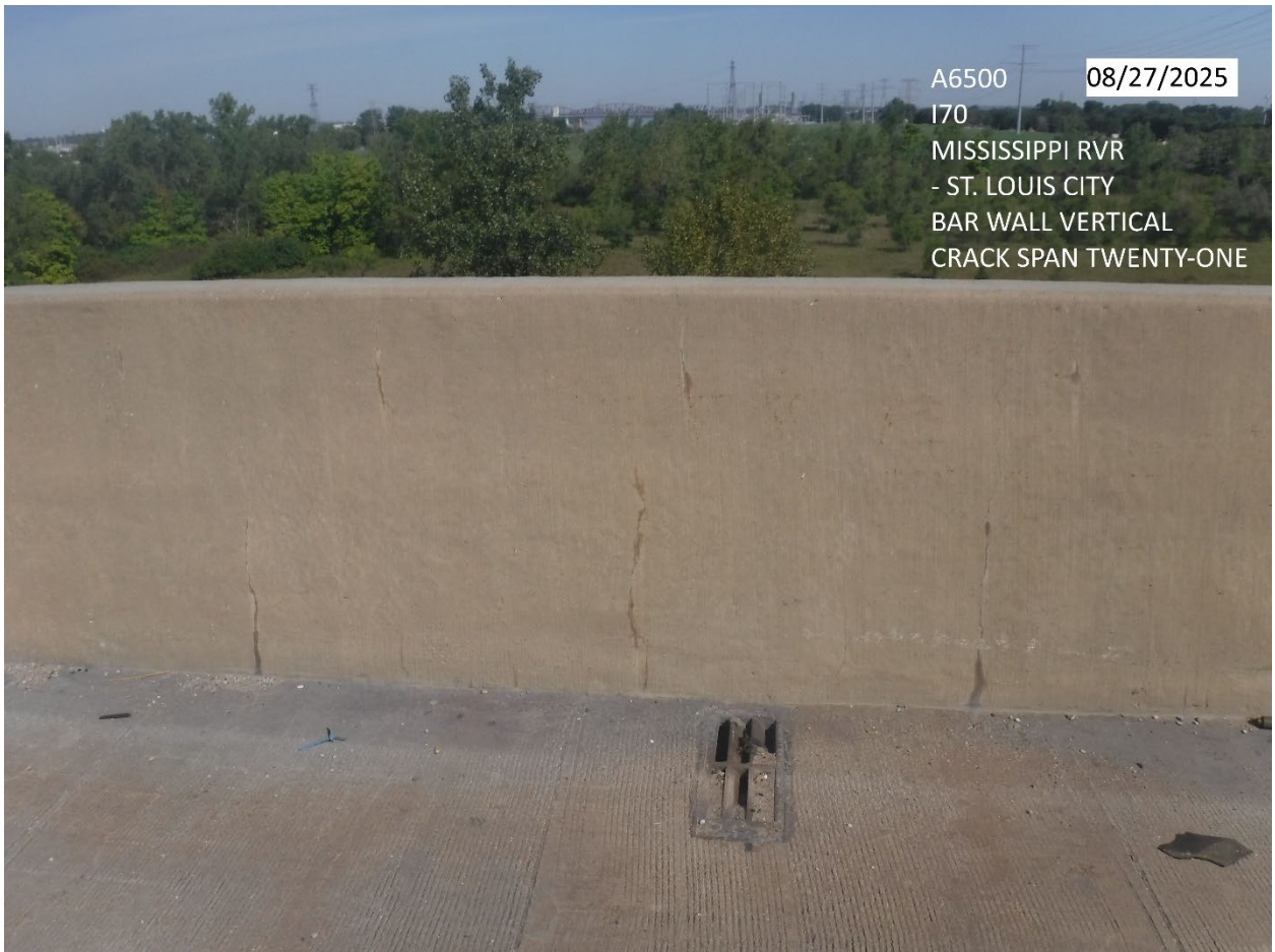
A6500 08/28/2025 I70 MISSISSIPPI RVR - ST. LOUIS CITY SPAN 10 NORTH BARRIER DETERIORATION
