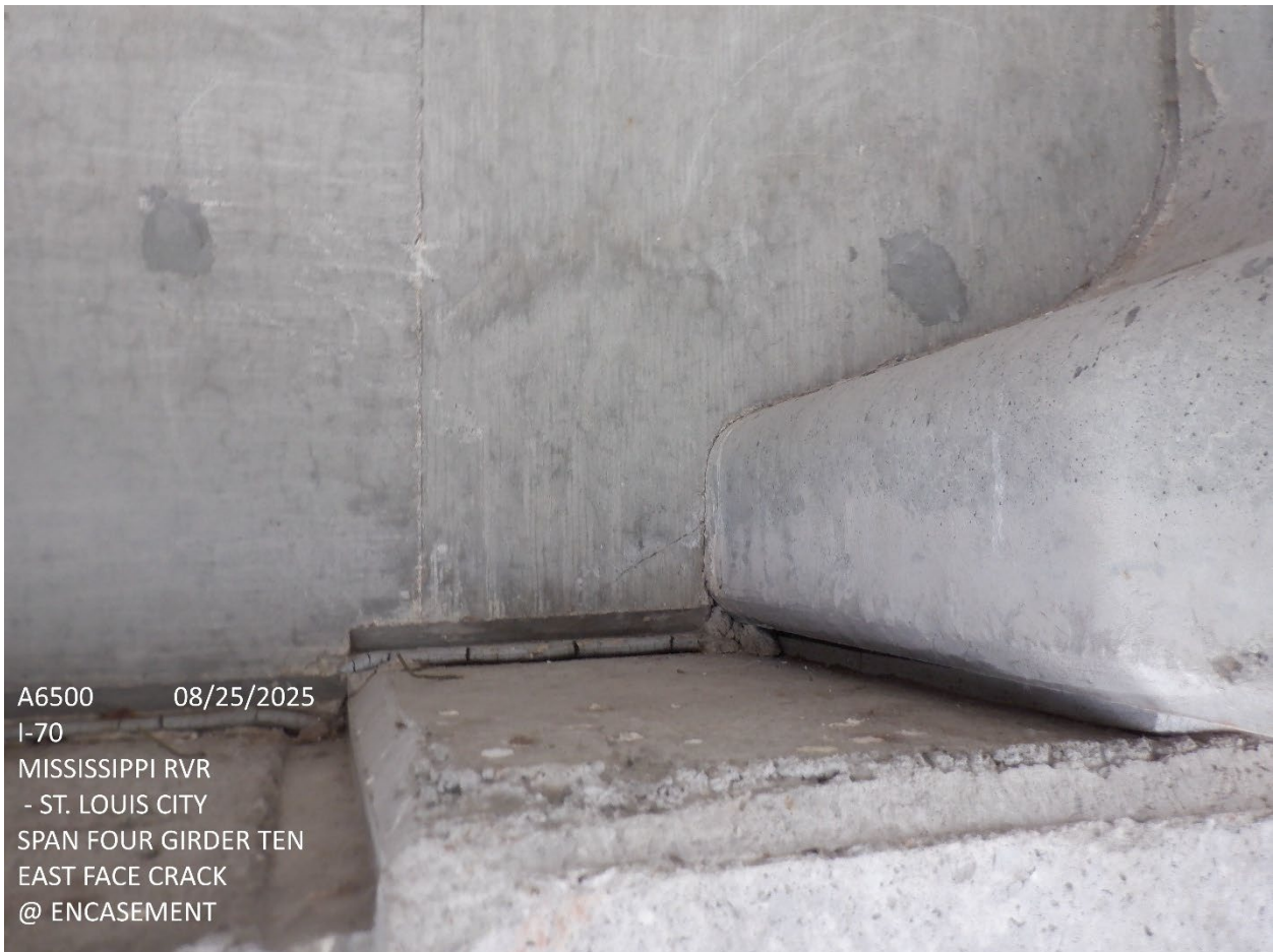
A6500 08/25/2025 I-70 MISSISSIPPI RVR - ST. LOUIS CITY SPAN FOUR GIRDER TEN TOP FLANGE CRACK WITH EFFLORESCENCE
