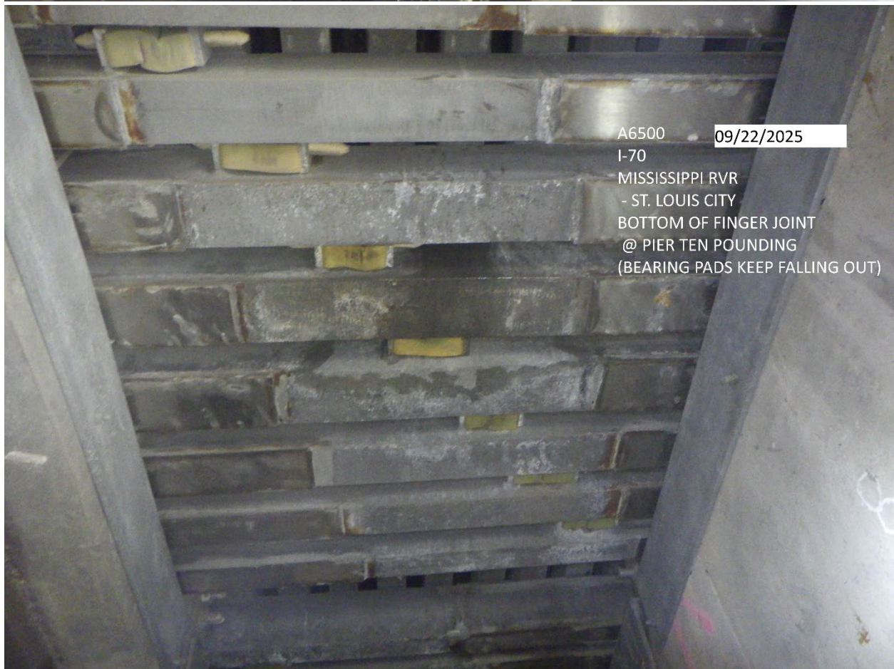
A6500 09/22/2025 I-70 MISSISSIPPI RVR - ST. LOUIS CITY BOTTOM OF MODULAR JOINT AT PIER TEN LOOKING SOUTH
