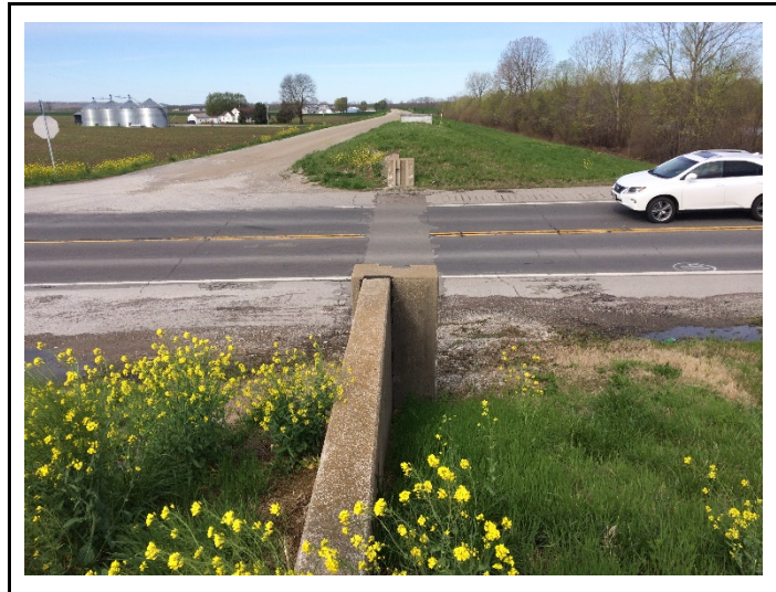
Figure 1-6. Gap in Bois Brule Levee at Route 51
