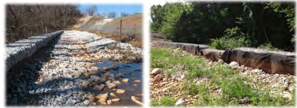
Rock / Mesh Control Fence
