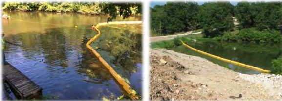
Sediment Drop Curtin
