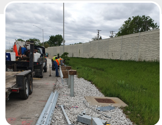
Project: Stan Musial/Veterans' Memorial Tollway, Roadway, and Bridge Rehabilitation I-55 (M.P. 12.3) to Army Trail Road (M.P.29.8) CM
