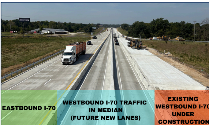
Westbound I-70 traffic between Callaway County Routes M (mile marker 144) and J (mile marker 137) has been shifted into the median while crews reconstruct the existing westbound lanes. The new lanes within the median will eventually serve as the third lane and inside shoulder of both eastbound and westbound I-70.
