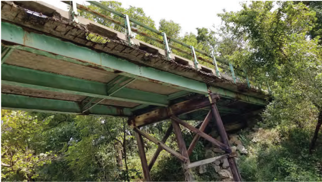
PHOTO 7 - DECK DETERIORATION (WEST FASCIA, MIDDLE SPAN)
