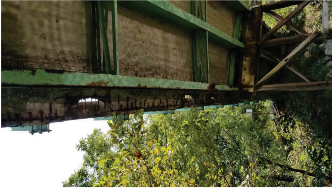
PHOTO 5 - DECK DETERIORATION (EAST OVERHANG, MIDDLE SPAN)
