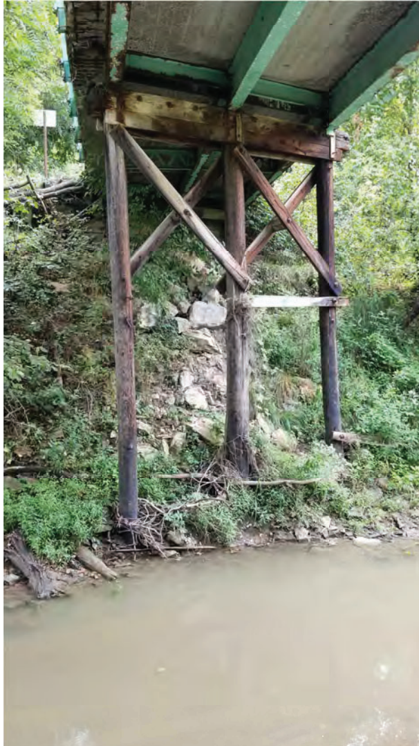
PHOTO 13 - BOWED, SPLIT PILES MISSING BRACING (SOUTH PIER)
