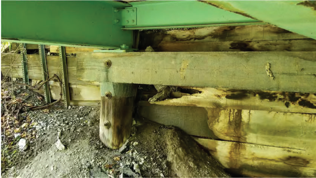
PHOTO 11 - ROTTED AND WEATHERED TIMBER BACKWALL (NORTH ABUTMENT)
