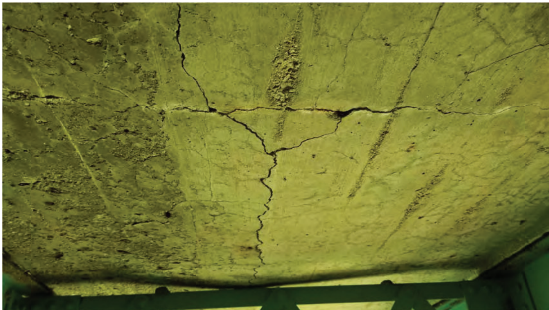
PHOTO 8 - DECK FAILURE (EAST BAY, NORTH SPAN)
