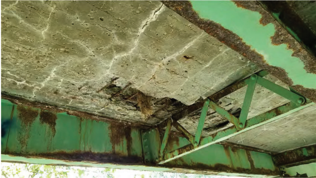
PHOTO 3 - LOCAL DECK FAILURE (SOUTH SPAN, WEST BAY)
