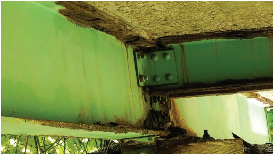
PHOTO 10 - RUST, CORROSION (EAST STRINGER, SOUTH END - NORTH SPAN)
