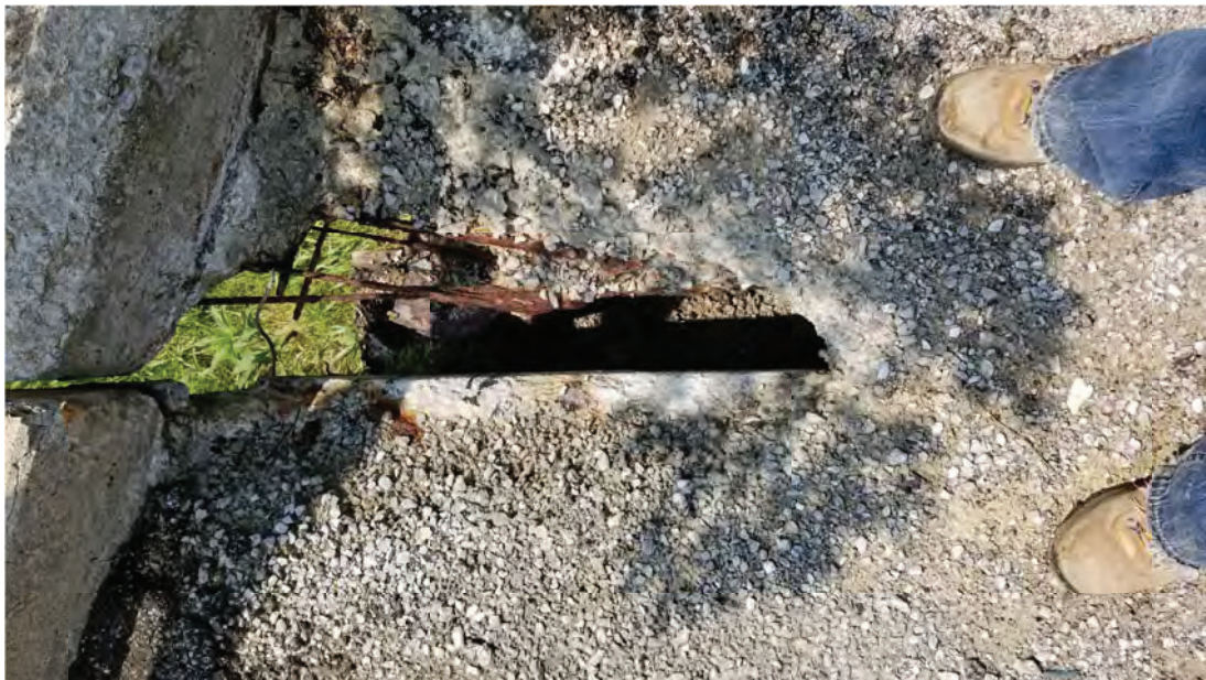
PHOTO 4 - DECK SPALL (OVER NORTH PIER)
