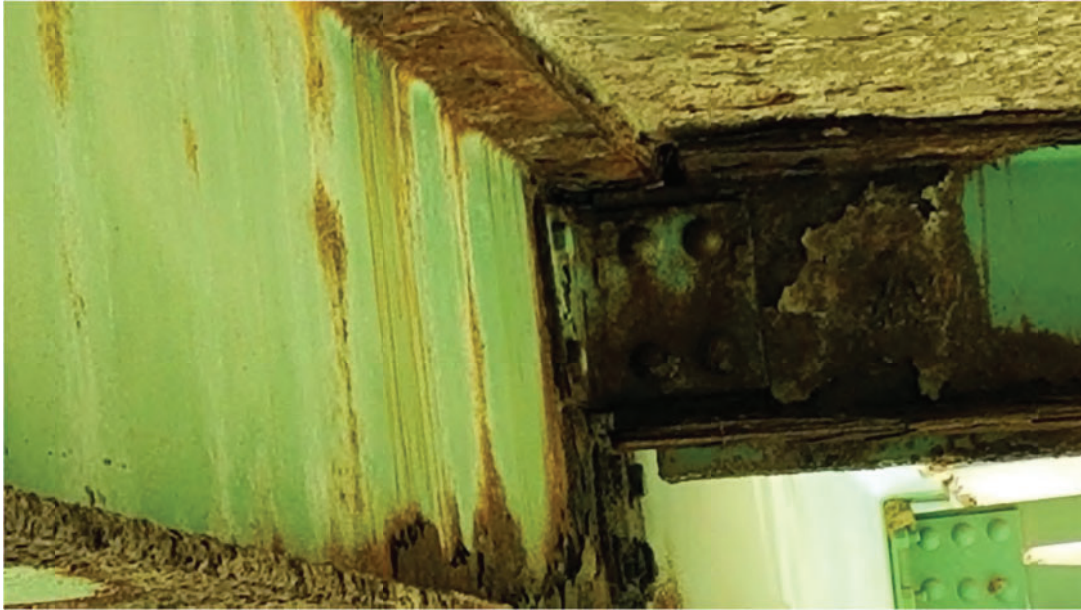
PHOTO 9 - STRUCTURAL STEEL, RUST & CORROSION (MIDDLE STRINGER, SOUTH END - NORTH SPAN)
