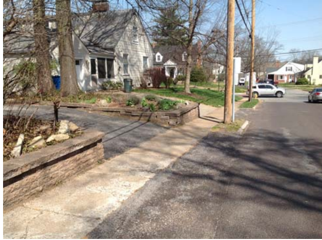
Photo - #1 Non ADA sidewalk and in poor condition, slight rutting, longitudinal cracking
