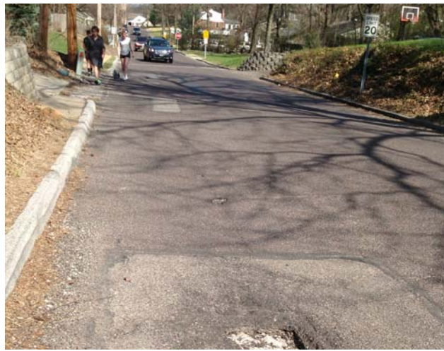
Photo - #3 No sidewalk, rutting in wheel path, utility patchwork, pot holes
