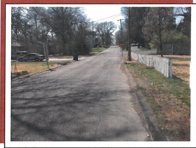
Rutting in the wheel path.
