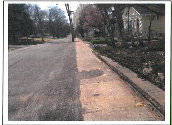
Sidewalk is not A.D.A. compliant.
