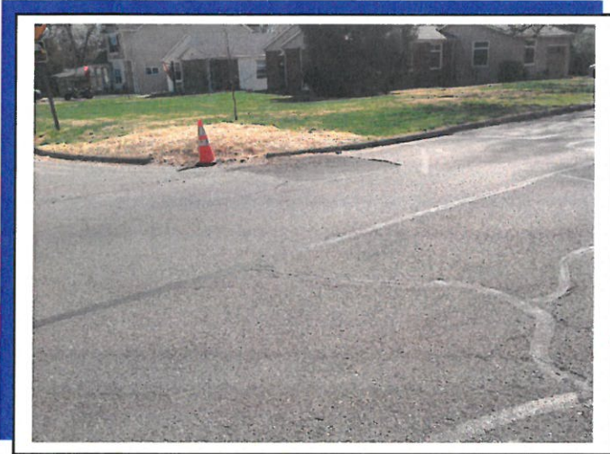
Utility patchwork and mild cracking.
