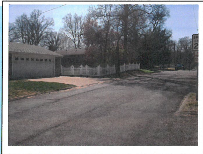
Longitudinal cracking and slight rutting.
