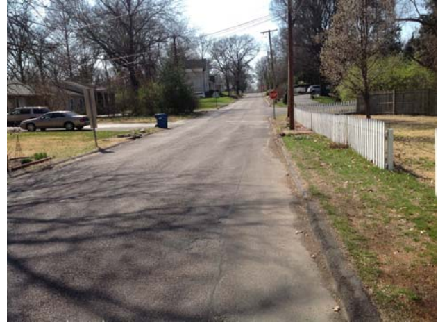
Photo - #2 No sidewalk, rutting in wheel path, utility patchwork, mild cracking
