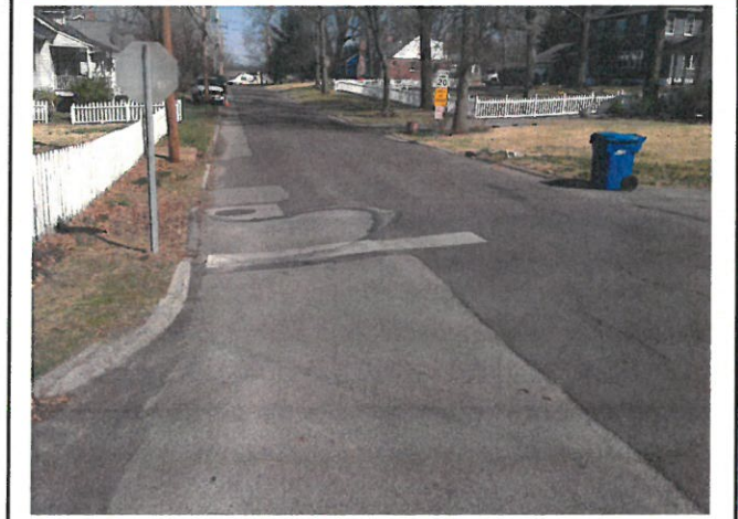
Utility patchwork as well as rutting and shoving.
