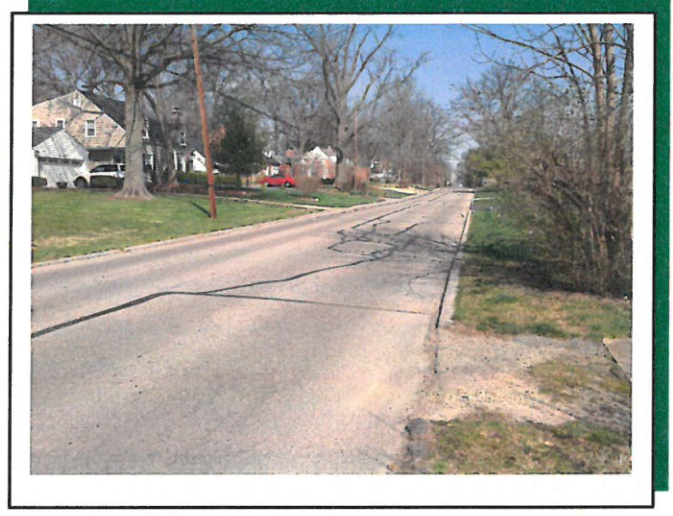
Longitudinal cracking and faint alligator cracking.
