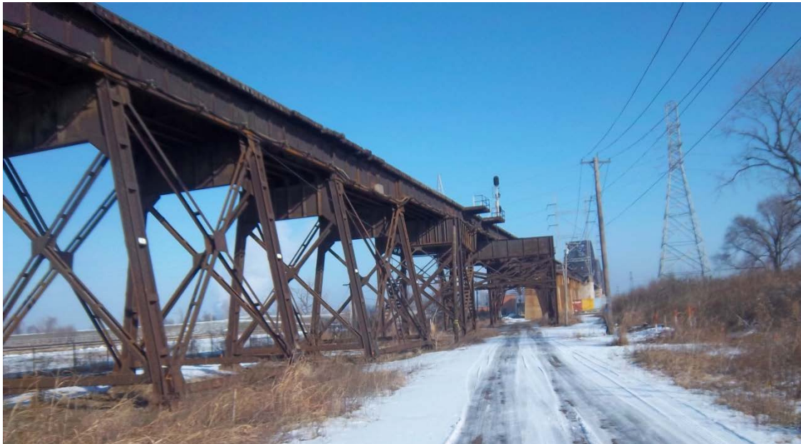
Looking east along Ferry Street at south side of West Approach toward Pier W6 and main river spans.
