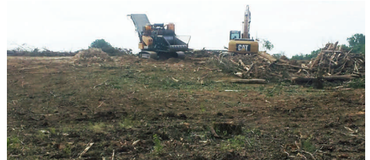
Hansen's Tree Service removing trees along the Route 364/Page Phase 3 project last year. Those trees were then recycled into mulch.
