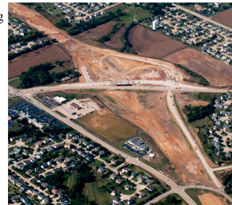
Aerial view of new Bryan Road with the extension of Route N (on right).
