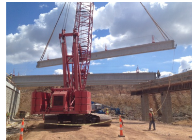
Crews place the bridge girders (support beams) for the new Bryan Road bridge over the future lanes of Route 364.
