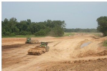
Crews move dirt from Gutermuth west building the roadbed for new Route 364.
