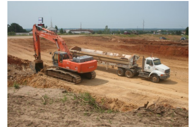
Excavation continues at Bryan Road. Trucks are hauling the dirt to the east side of Route
