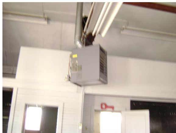
Overhead Heating Unit
