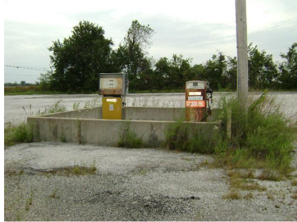
Gas Pumps/Fuel Containment Area
