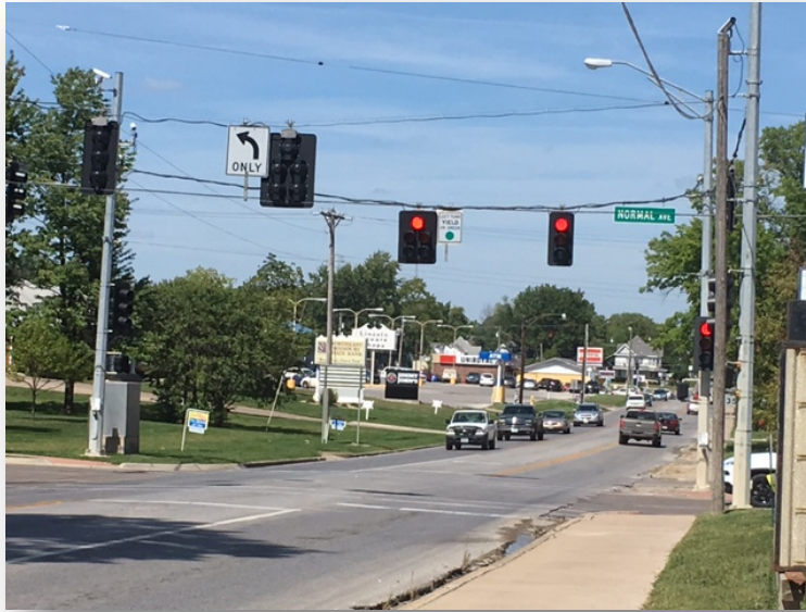
Figure 6: Many of the existing signals on U.S. Business 63/Baltimore Street in Kirksville are temporary
