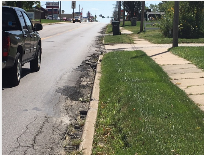
Figure 7: Continuous resurfacing of U.S Business 63/Baltimore Street over multiple decades has eliminated much of the capacity of the drainage system in Kirksville
